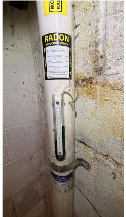
Existing radon mitigation pipe and U-tube manometer. The gauge confirms suction, not the actual radon level.
