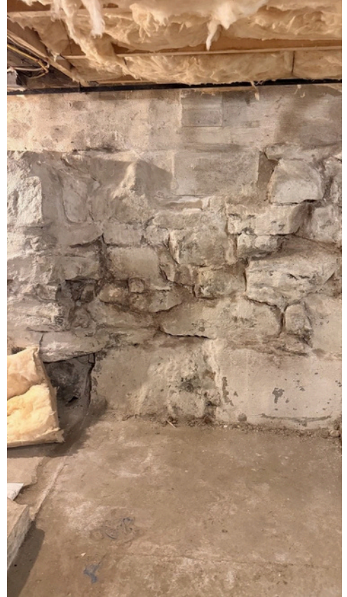
Original stone foundation showing extensive previous patching and repair work.
