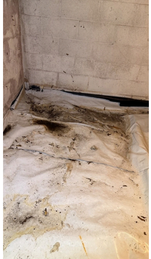
Existing exposed floor membrane showing staining, contamination and loose/wrinkled installation.
