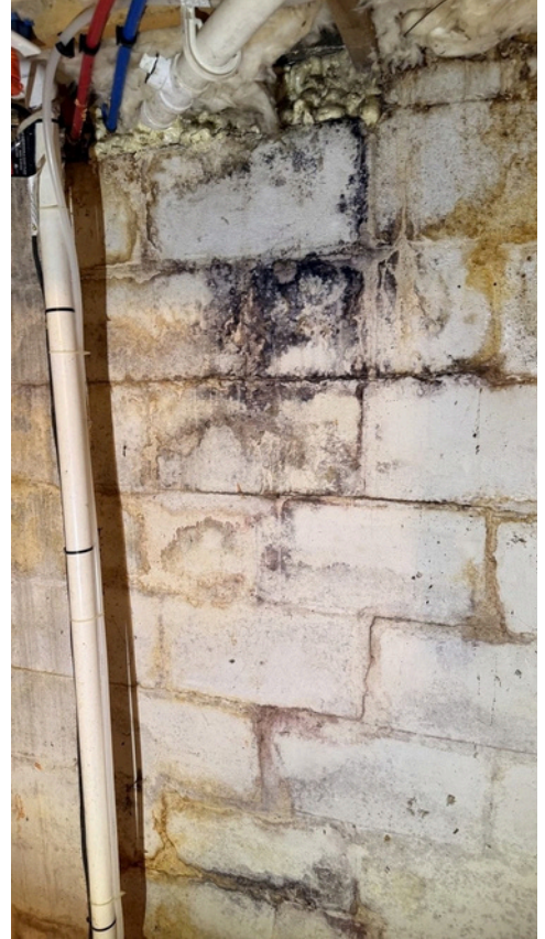
CMU wall with DRYLOK, moisture staining and dark growth/staining consistent with prolonged damp conditions.
