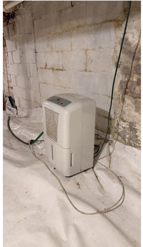
Existing portable dehumidifier in the basement near moisture-affected CMU and stone foundation areas.
