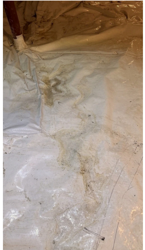
Current exposed membrane over crushed stone. Recommended replacement is a sealed sub-slab membrane protected beneath a concrete floor.
