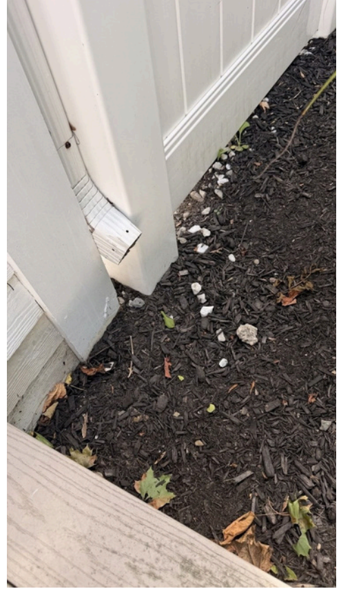
Downspout terminating directly at the foundation and discharging into the stone adjacent to the house.
