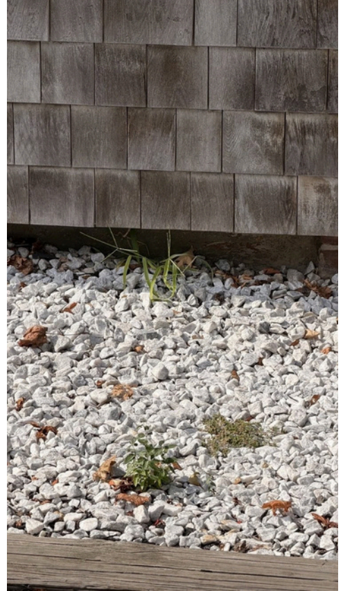
Very limited foundation exposure above exterior grade with crushed stone directly adjacent to the building.
